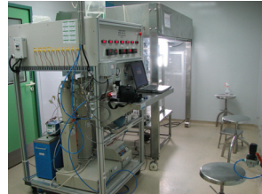
GMP CAN-BD powder manufacturing equipment installed at the Serum Institute (Pune, India) for the production of myo-inositol based inhalable dry powder measles vaccine for the NHP toxicity study and Phase I clinical trial.
